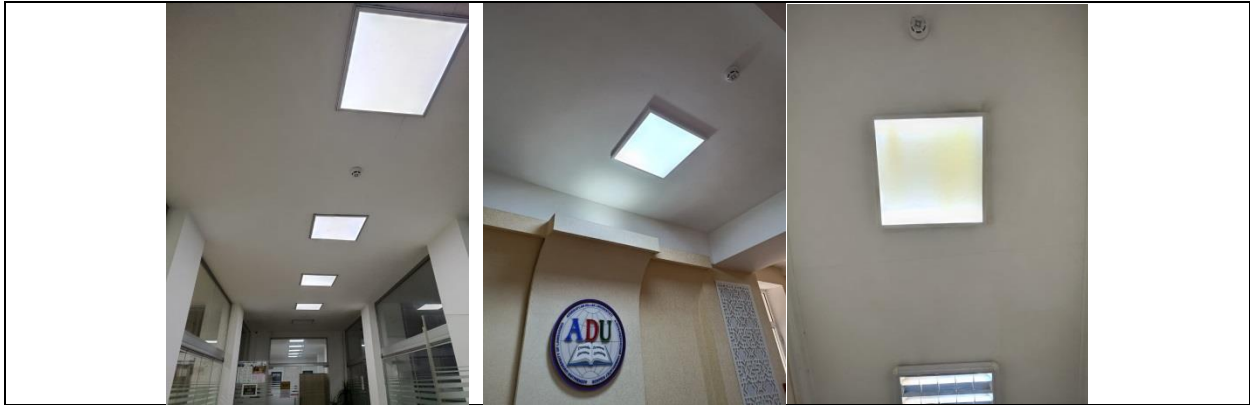
Example of Energy Efficient Appliances Usage: Use of LED lighting and lamps with light detection (Azerbaijan University of Languages)
