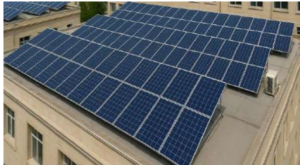
Example of Roof Mounted Solar Panels (Azerbaijan University of Languages, Azerbaijan)
